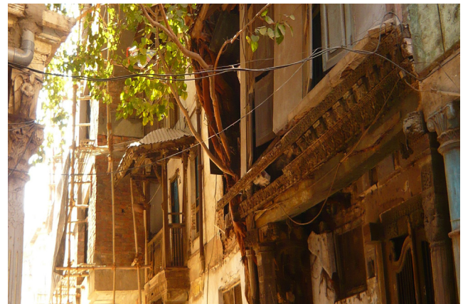
Distress in traditional structures in Ahmadabad; Image Credit: Khushi Shah, 2011
